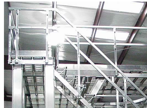
Eighteen feet high aluminum platform with stair assembly.
